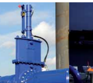
VALVES A dredge valve or non-return valve can be placed in the discharge piping.
